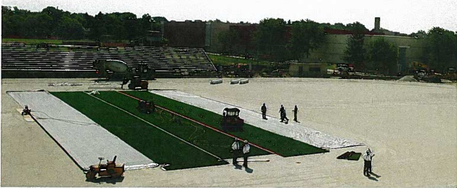
A view of the new Barrington Community Stadium from atop the home fans' grandstand, looking east across the field as the new turf was laid.
