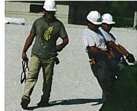
Workers unrolled sections of FieldTurf®, which were then sewn together and anchored to the playing surface of the new stadium.
